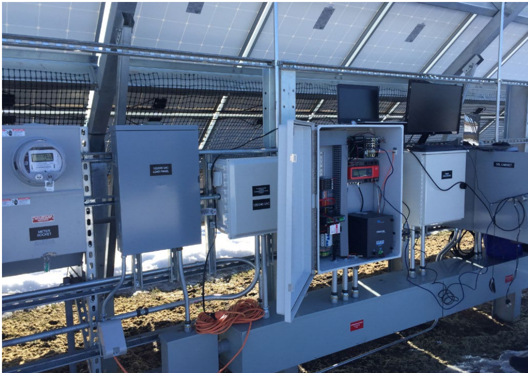
Figure 8-5. Bozeman Solar Microgrid Container Boxes and Controllers
